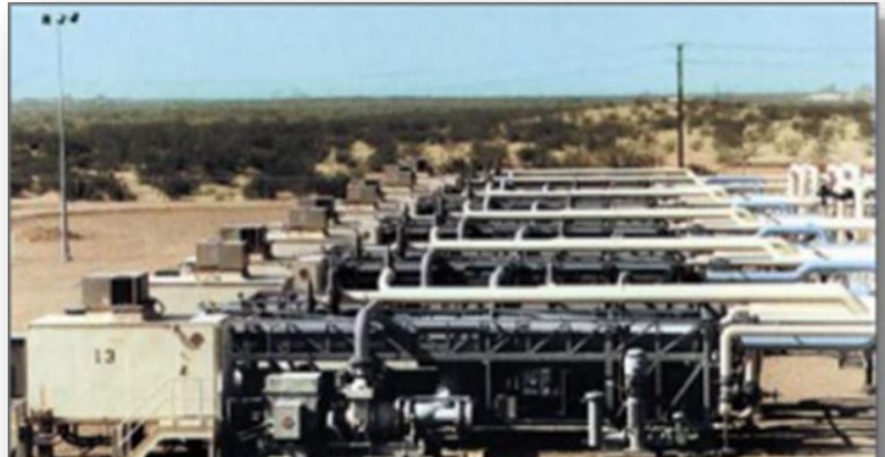
1986: 30 MW Ormes 1 Geothermal Plant in East Mesa, California
